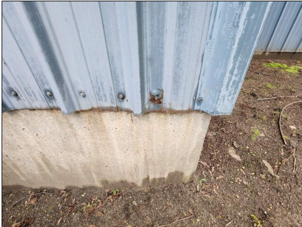
Rusting Metal Siding and Fasteners.
