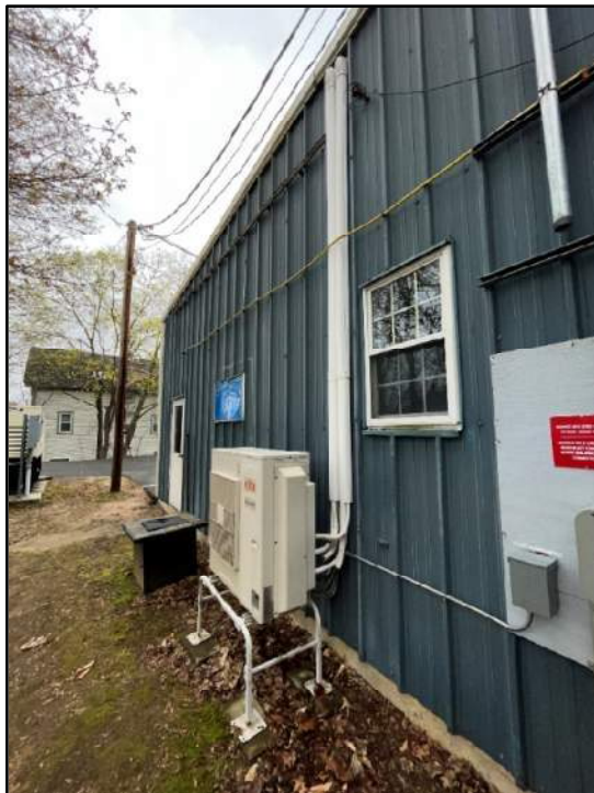
Firehouse condensing unit for all the interior heat pump units.
