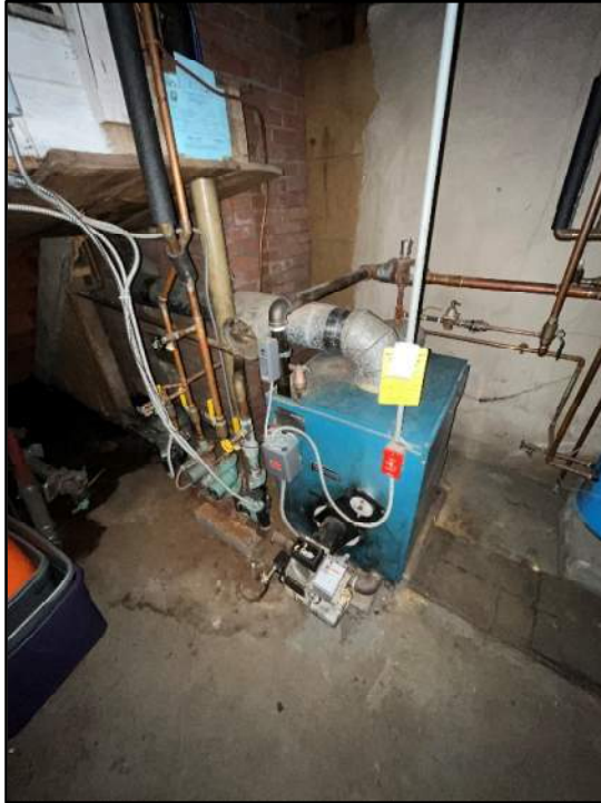
The residence house's existing boiler is located in the basement.
