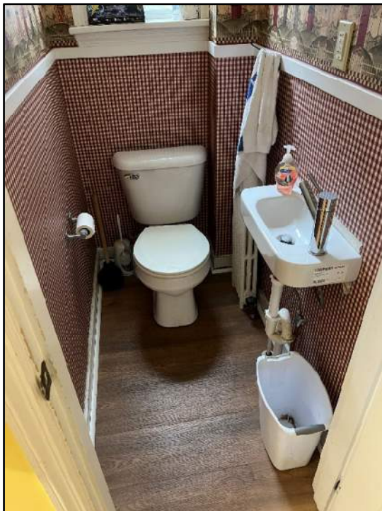
Residence house floor-mounted flush tank toilet, sink, and existing hot water radiator.
