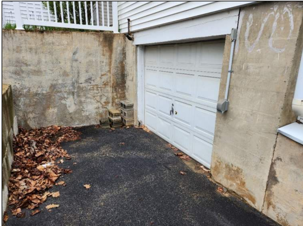
Office Overhead Door.
