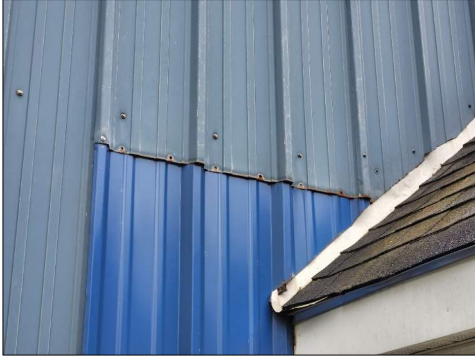
Patch in the Metal Siding.
