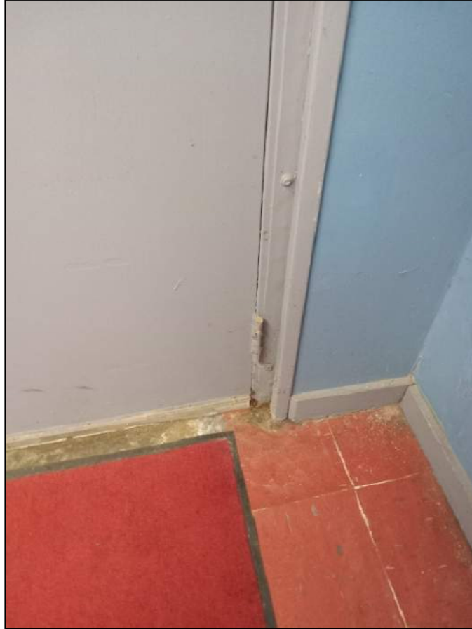
Exposed Concrete Between Finish Flooring and Exterior Door Threshold.
