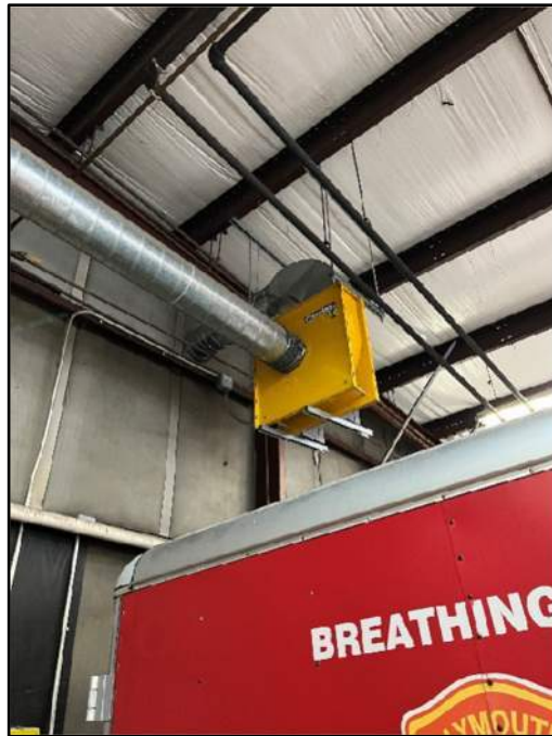
Firehouse garage exhaust system exhausting to the outside.
