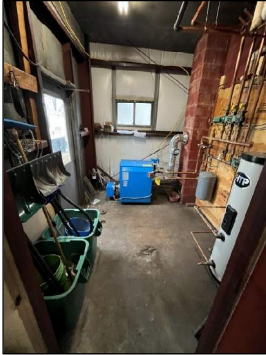
Firehouse boiler room set-up with boiler, expansion tank, hot water tank, & distribution pumps.
