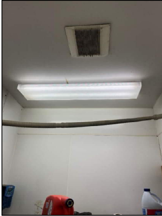
Firehouse exhaust from laundry room discharging to gooseneck on the roof.
