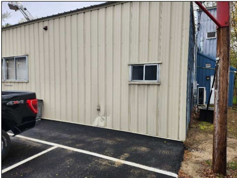
Dented Metal Siding.
