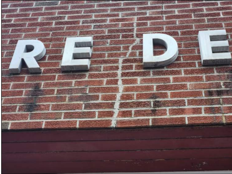
Crack in Brick Veneer.
