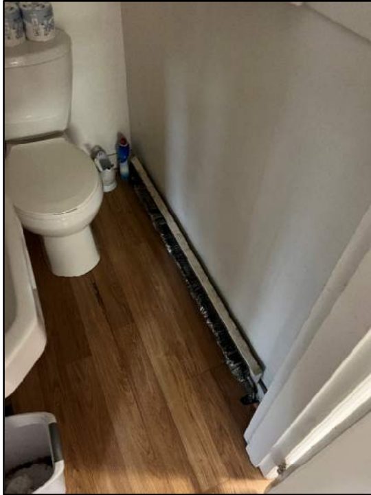
Damaged fin tube baseboard heater missing a protective cover in the residence house.
